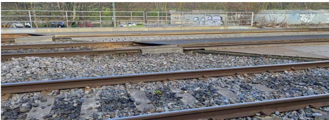
Damage to the transition zone at the rail bridge over Sarsfield Road in Dublin.
